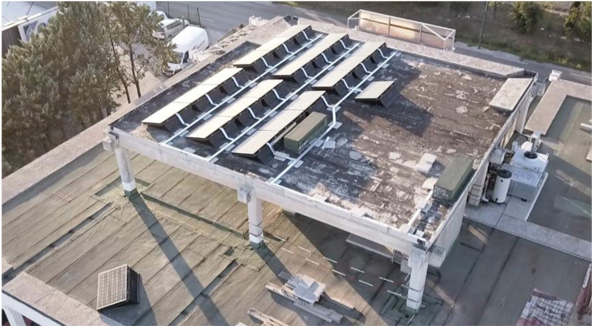
Fig. 3: Global view of 18 mono-crystalline PV plant and chiller unit on ATISYS roof
