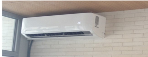
b) PV - Air conditioner: internal unit
