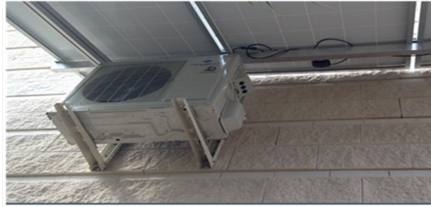
a) PV - Air conditioner: external unit
