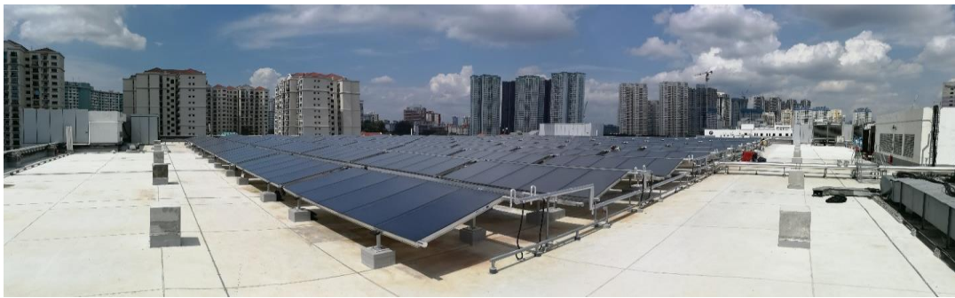
Fig. 6: Panorama view of 2472m 2 collector area installed at IKEA.
