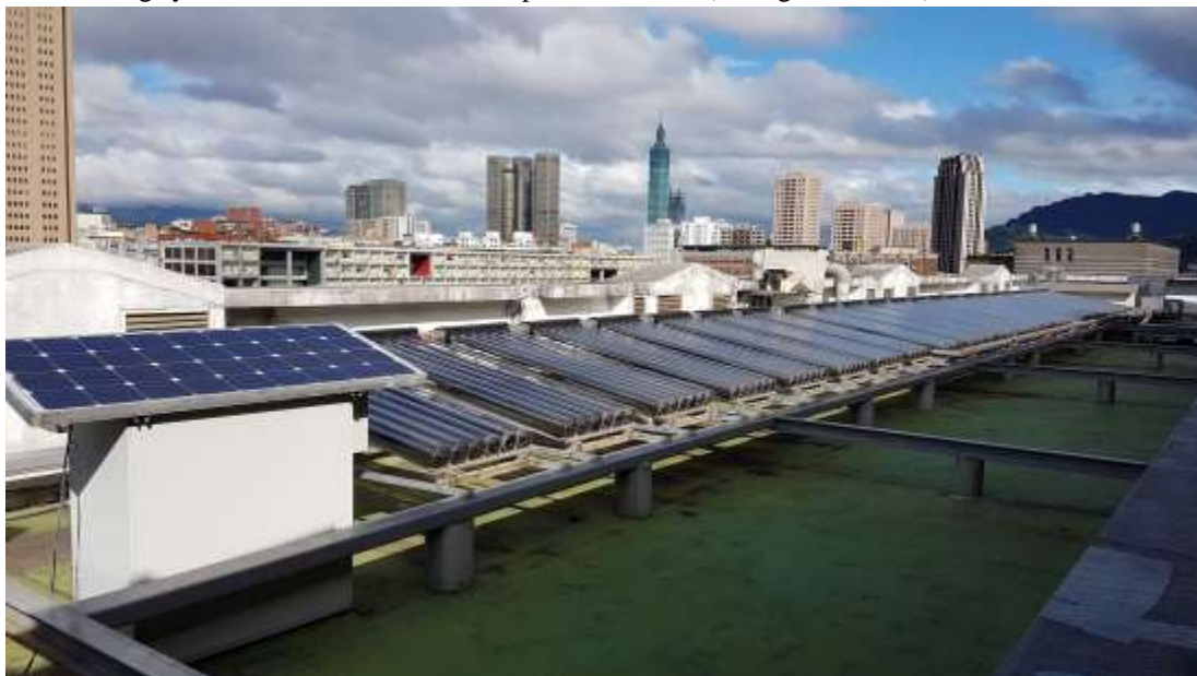
Fig. 2: Vacuum-tube solar collector of SACH (Huang et al., 2012).
