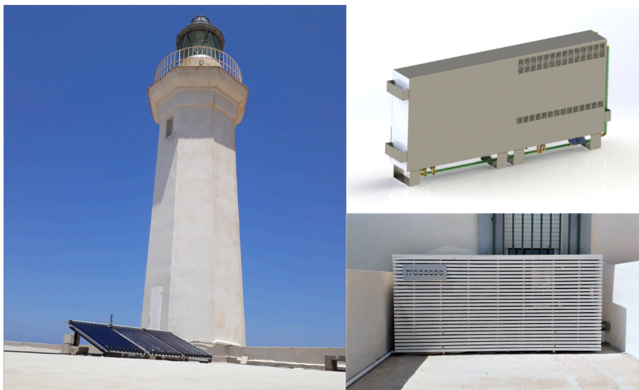
Fig. 2: Picture of the freesco system for facade integration monitored at ENEA Research Center in Lampedusa
