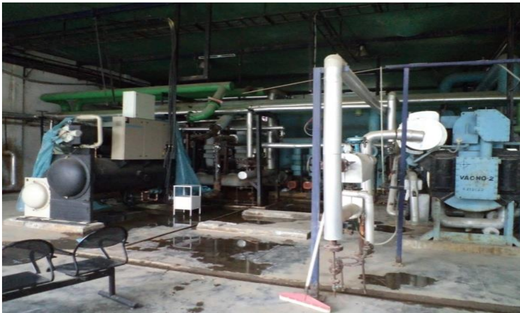
Figure 8 Vapor Absorption Cooling (VAC) machine
