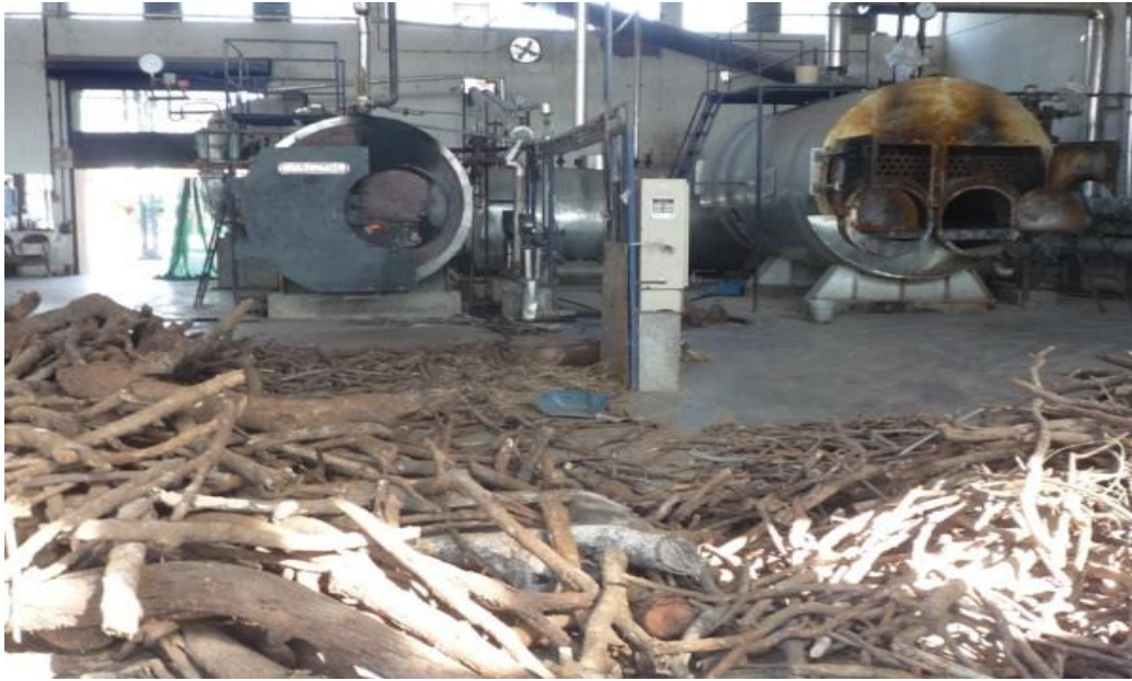
Figure 9 Biomass fired boiler from the site
