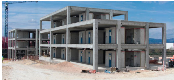
Fig. 7: Reinforced concrete framed building construction (“Reinforced concrete portal frame / prestressed concrete - Pujol,” n.d.)
