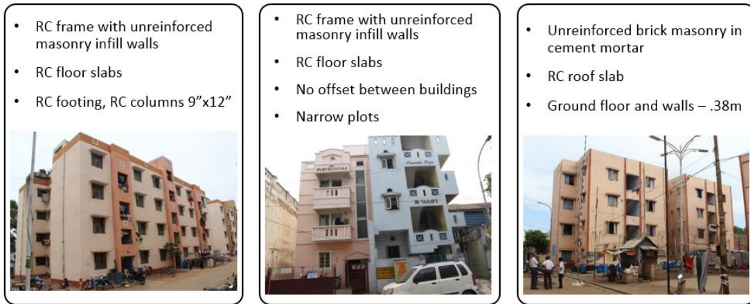
Fig. 6: Building typologies in the state of Tamil Nadu (National Disaster Management Authority, 2013)
