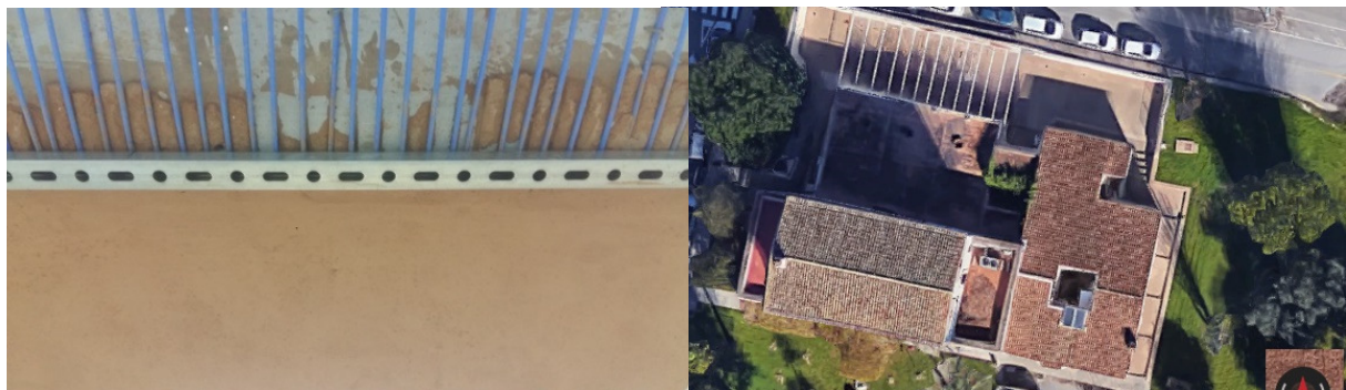
Fig. 1: View of the capillary radiant system and top view of the seminar room
