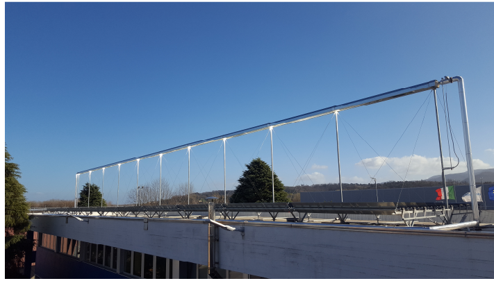
Fig. 1: FLCM Solar Plant in Lucca, Italy.
