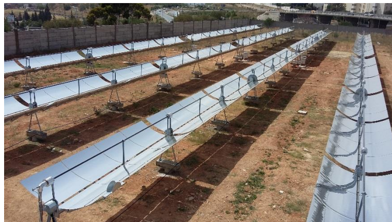
Fig.6: Solar field of REELCOOP plant
