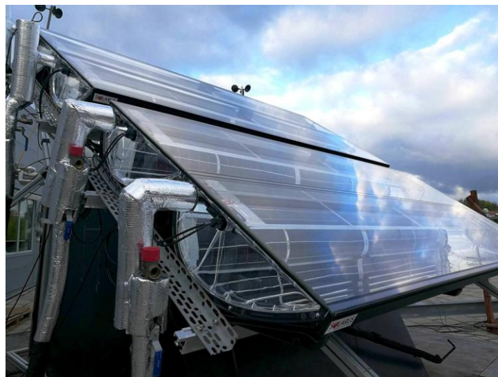
Figure 5: Rooftop collector mounting stand.
