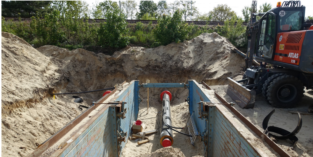
Figure 3: Installation of the heat pipeline to tunnel under the rail trail (picture: Solites, 16.05.2019)
