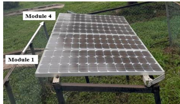
Fig. 2: Picture of the installed system
