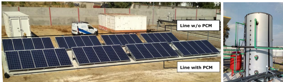
Fig. 1: Physical arrangement of the solar field (left) and stratified storage tank (right).
