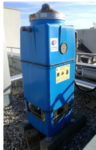
Fig. 5: Wet cooling tower on the roof-top of the University of Applied Sciences Upper Austria
