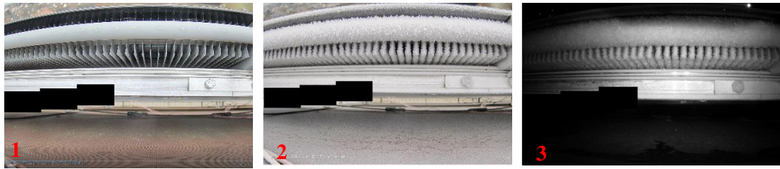
Fig. 6: Ice formation under the PVT collector field (back side of the PVT – fins surface)
