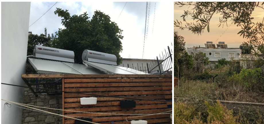
Fig. 6: Solar siphons in the garden (left) and on the roof (right)
