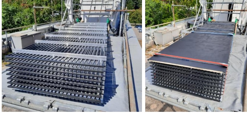
Fig. 1: Illustration of the two variants investigated, left: uncovered (variant 1), right: covered (variant 2)
