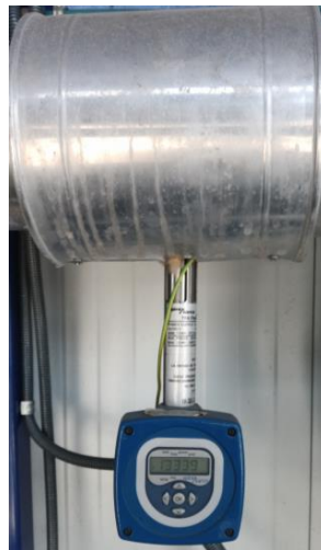
Fig. 3: Steam mass flow meter installed at the extraction side of the skid
