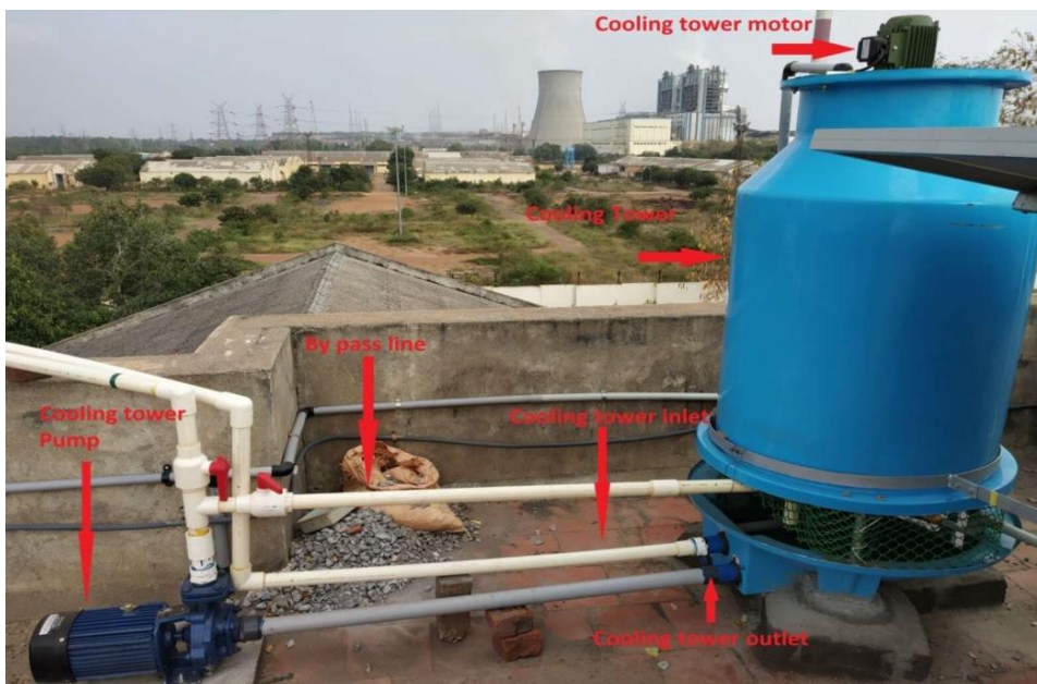
Fig.7: Cooling tower with cooling water pump
