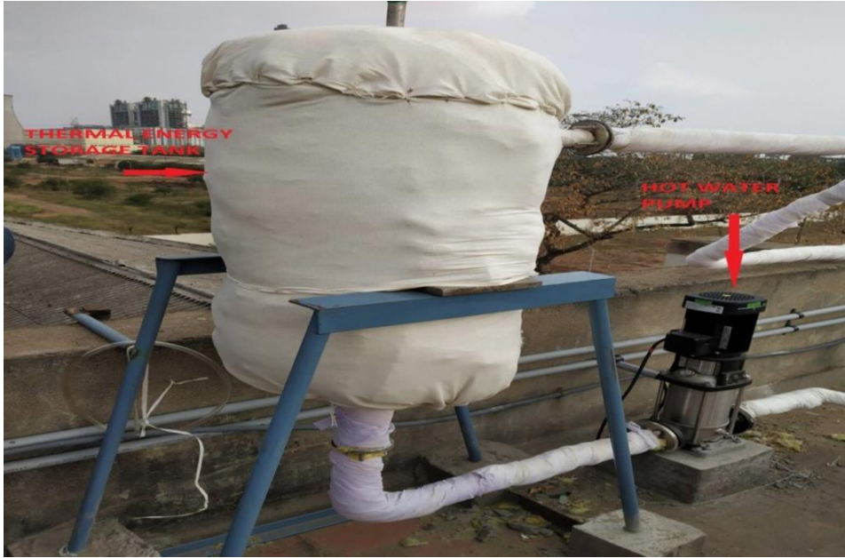
Fig. 6: Sensible thermal storage tank with hot water pump
