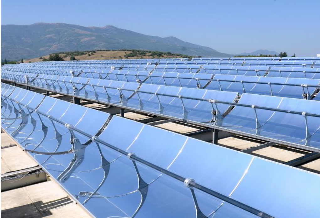
Fig. 3: SOLITEM PTC 1800 Parabolic Trough Collectors in the project location in Turkey
