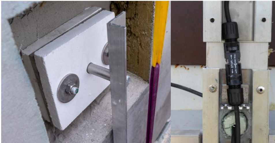
Fig. 4: Left: Facade anchors with thermal separation via calcium-silicate plates (Stark Ingenieure). Right: Strain relief within the pilaster strips
