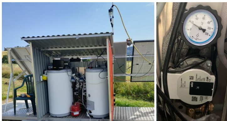
Fig. 3: Water tanks and hydraulic pump
