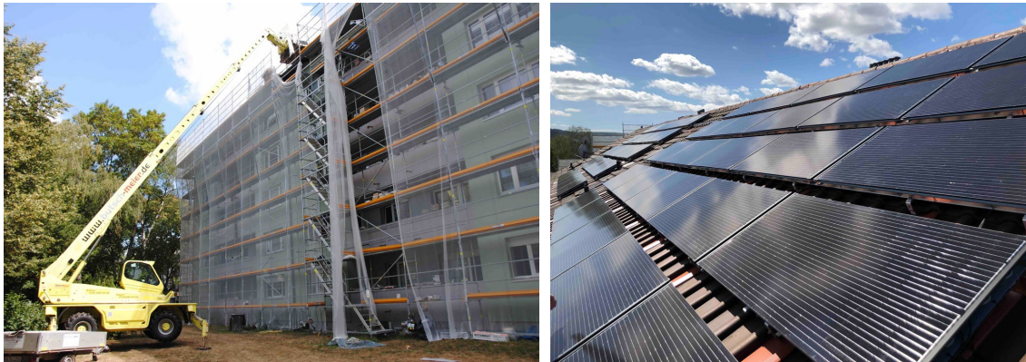
Fig. 6: Transport of SOLINK collectors to the roof of the apartment building (left). SOLINK collectors installed on the roof (one half of the roof and one half of the field) (right)
