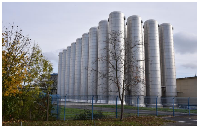
Fig. 2: Slim hot water storage tanks, four times nine storage tanks in series, Chemnitz (Germany) district heating supply, operator eins/inetz
