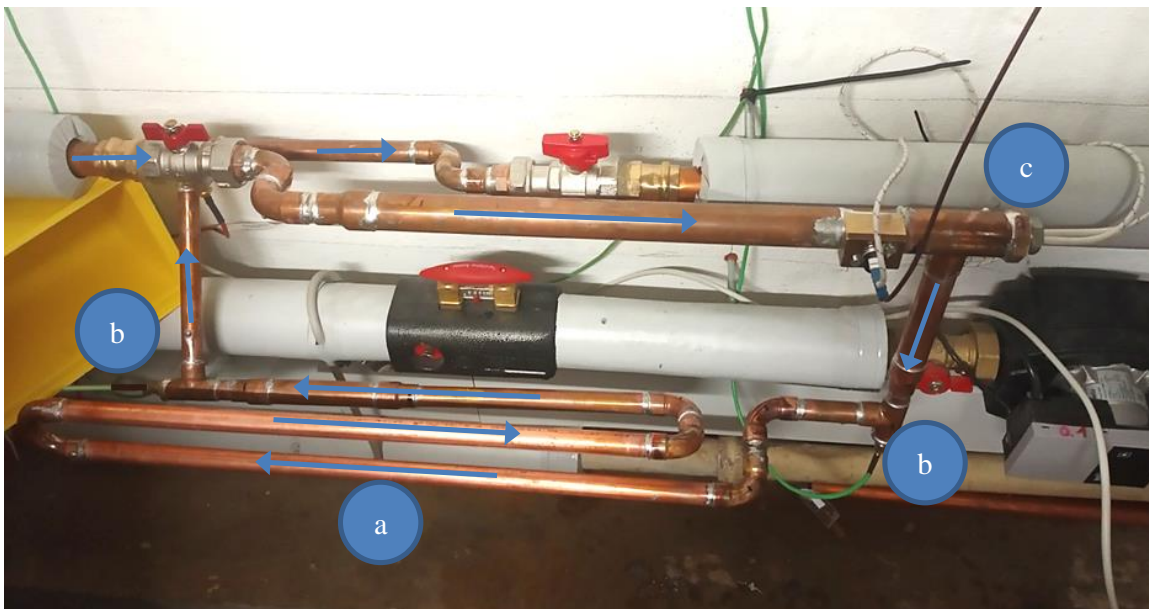
Fig. 4: Measurement track (a) with temperature sensors (b) and electrical heating element (c); Note: Shown without thermal insulation for better clarity
