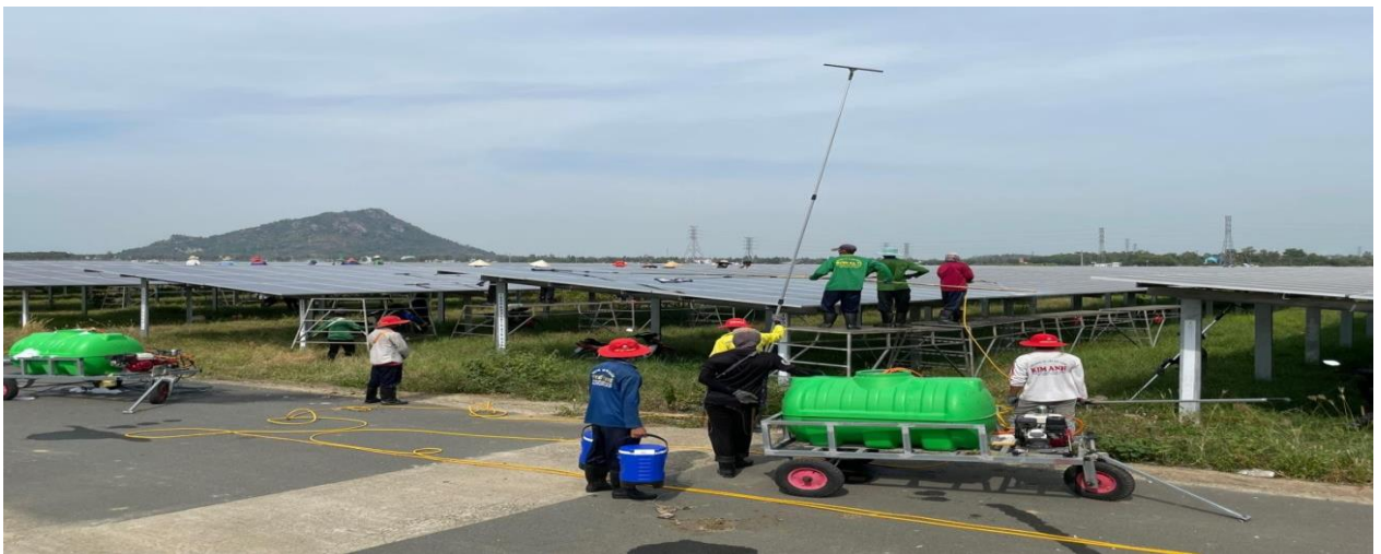
Fig.2 : Traditional cleaning of panels
