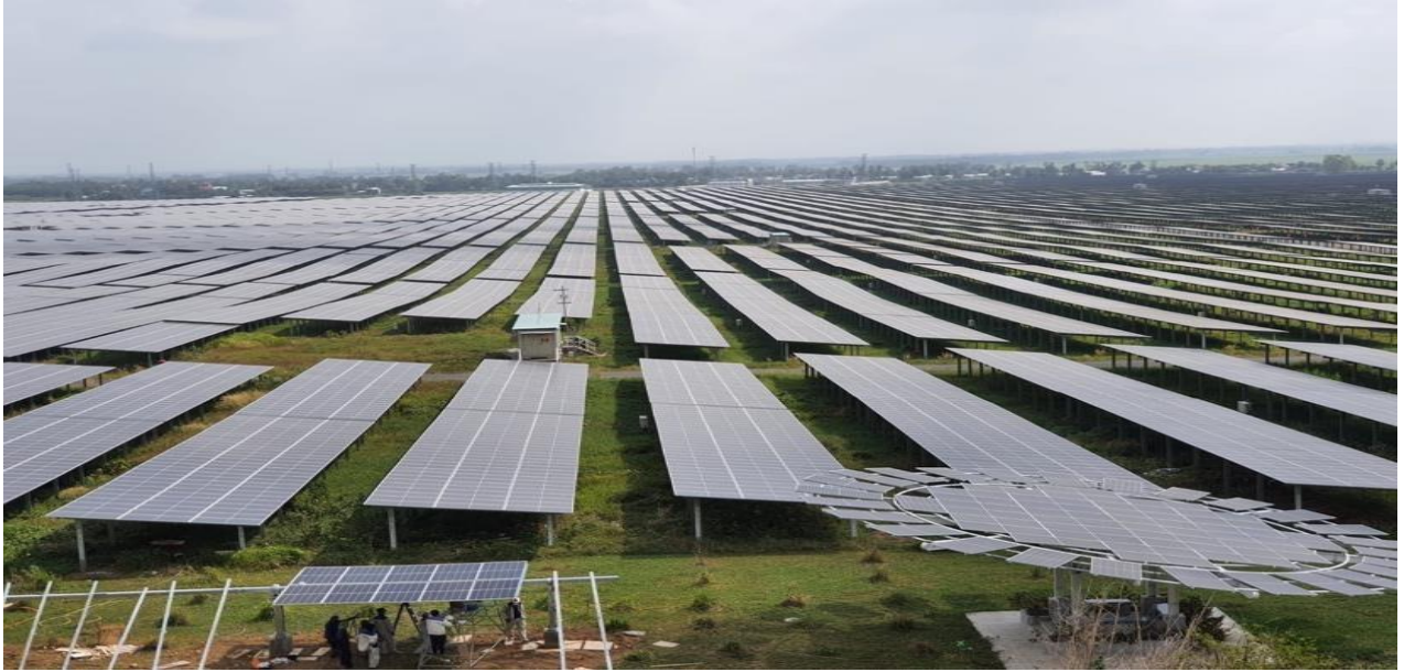
Fig 1 : Sao Mai PV1 solar farm at vietnam
