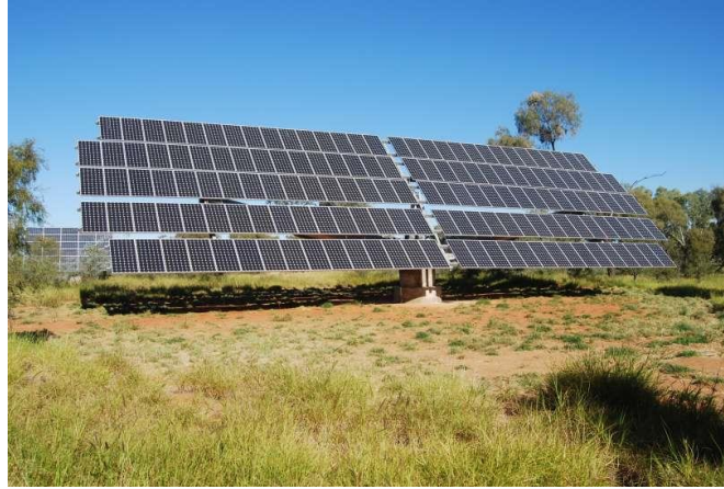
Fig. 4: The dual-axis tracker 26.5kW photovoltaic system of site 2 of the Desert Knowledge Australia Solar Centre (DKASC-2), in Alice Springs, Central Australia, working between August 24 th ,2010 to December 1st, 2012. Source: DKA.
