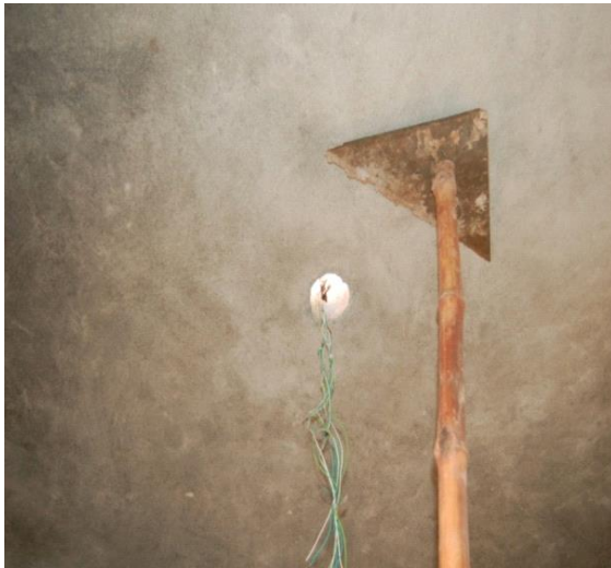
Fig. 9: Temperature sensors inserted in RCC ceiling
