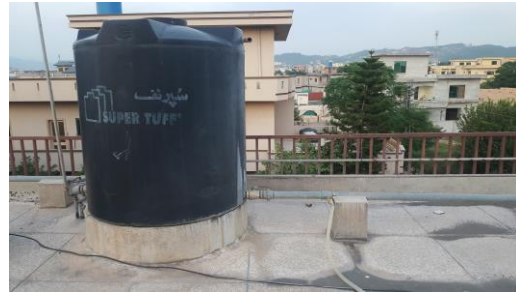
Fig. 4: Watering pipe connected to the overhead tank installed on the roof
