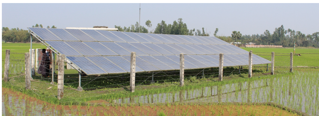
Fig. 6: IDCOL financed Solar Pump. 14.4 kW p solar array powering a 10 HP submersible pump irrigating 72 bighas (~24 acres) of rice for 25 farmers in Biral, Dinajpur. The SWP installation cost was BDT 3,500,000 (~US$41.1k)
