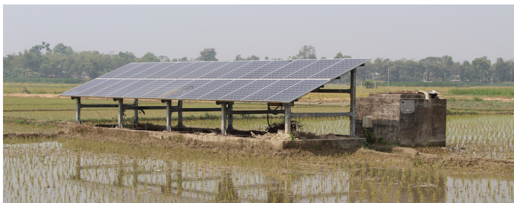
Fig. 5: KOICA financed Solar Pumping Project of BREB (5.16 kW p PV array in a rice field powering a 3.7 kW submersible pump providing 300 l/min in Singair, Manikganj.
