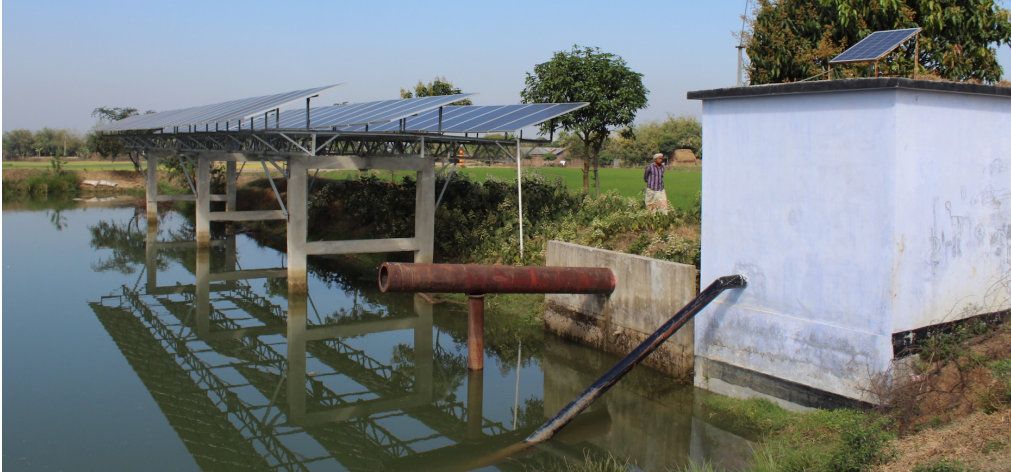
Fig. 7: BMDA 20.4 kW p SWP in Godagari, Rajshahi installed in 2016. System is operated with pre-paid cards. GoB funded installation R BDT 2,400,000 or about US$1.38 per W p , including additional cost of 1,500 meters of 10” PVC pipe for BDT 700,000.
