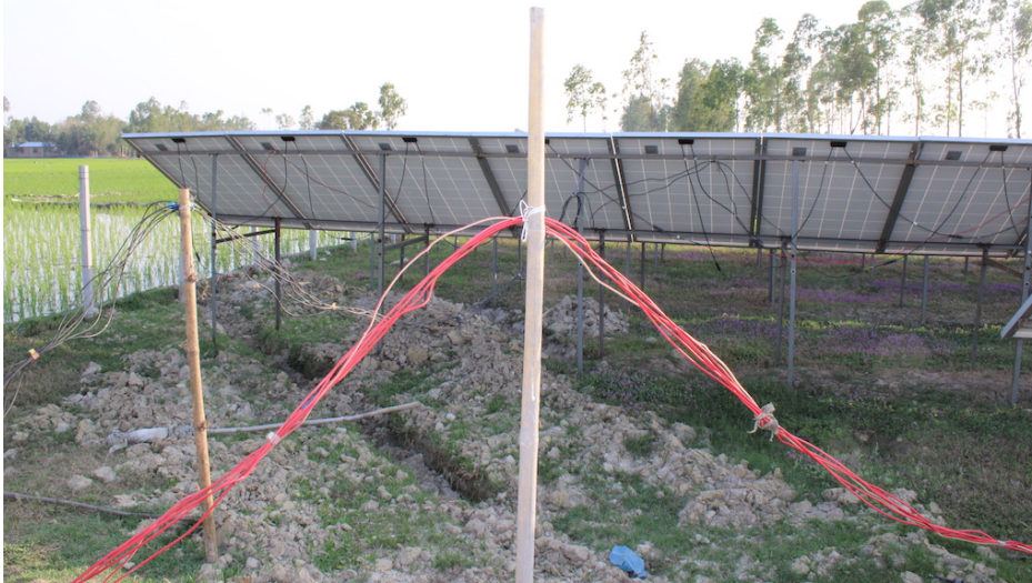
Fig. 11: Example of poorly installed wiring. Wires dangerously and carelessly scattered across the ground; the farmers came back and installed loose wires on the wooden posts. There is no ground and no array string fuse, presenting a significant electric shock hazard. This 30 kW p solar array powering a 20 HP submersible pump irrigating 48 bighas (~16 acres) of mostly boro and aman rice in Biral, Dinajpur. Water is sold to farmers at BDT 2,000 (US$ 23.50) per bigha.
