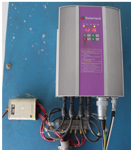
Fig. 13: A SWP project in Biral, Dinajpur with a inverter with no string fuses or SPD to help protect from power surges.
