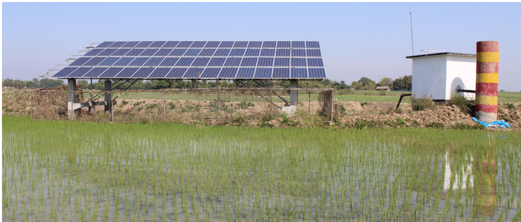
Fig. 8: BMDA 20.4 kW p (300 W p x 68) PV array used for rice irrigation in Rajshahi.
