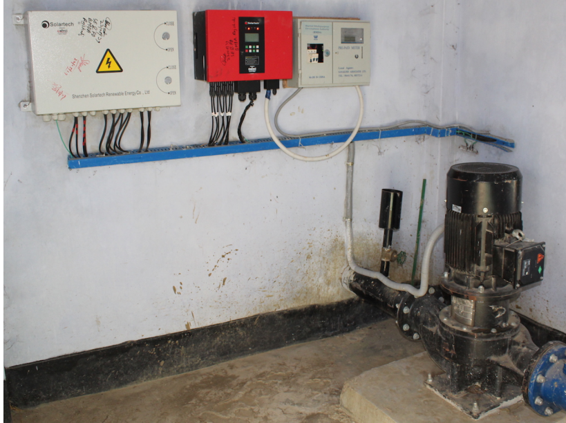
Fig. 9: BMDA Solar Surface Water Pumping System. MPPT Pump inverter with overcurrent protection for the DC strings. The pre-paid meter on the right uses AC circuit breakers. Note the green ground wire on the far left.
