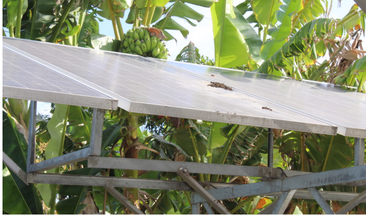
Fig. 10: Banana tress have grown taller than this array on the north side and partially shaded a PV string on this Biral SWP system causing module shading and related current drop and module hotspots that can lead to premature failure.
