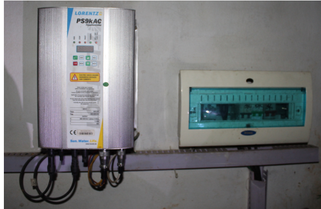
Fig. 12: Pump inverter used to power solar pump project in Setabjanj, Dinajpur. The system ran for 3 years and then a AC circuit breaker failed because it was inappropriately used in a DC circuit. It was replaced again with an AC circuit breaker in 2019 which can be expected to fail again.
