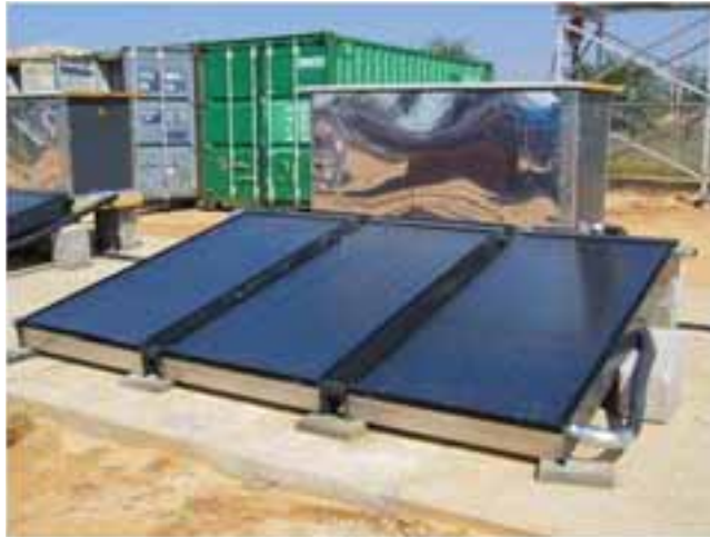
Fig. 1: Photograph of one of the six solar thermal desalination systems with heat recovery installed in Akutsima, Namibia.
