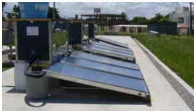
Fig. 2: Photograph of the three solar thermal desalination systems with heat recovery installed in Fortaleza, Brazil.
