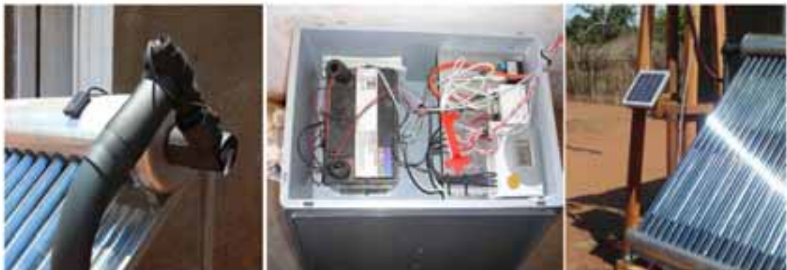
Fig. 5: The technical monitoring system of the solar water disinfection plant is shown in the pictures above (from left to right): Temperature and radiation sensors, logging equipment powered by a car battery and a PV-panel (pictures previously published in Komersmann/Frank 2009).
