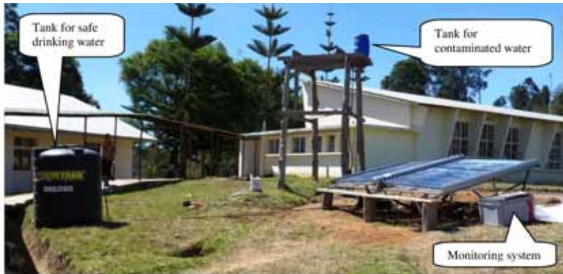
Fig. 4: The SoWaDis system installed at a university campus in Magamba/Tanzania.
