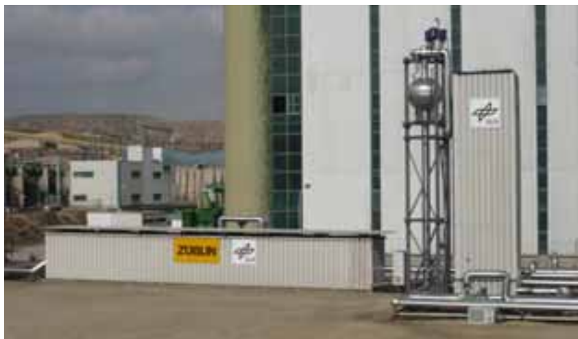
Fig. 10: Demonstration storage system with concrete superheater (left) and PCM-Storage (right) in the water/steam test loop at the power plant Litoral of Endesa in Carboneras, Spain
