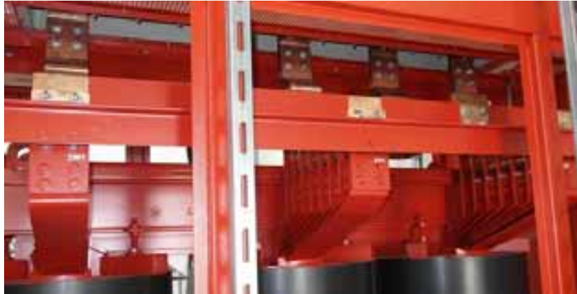
Fig. 11: Taps and adjustable star point at the secondary side of the tap transformer
