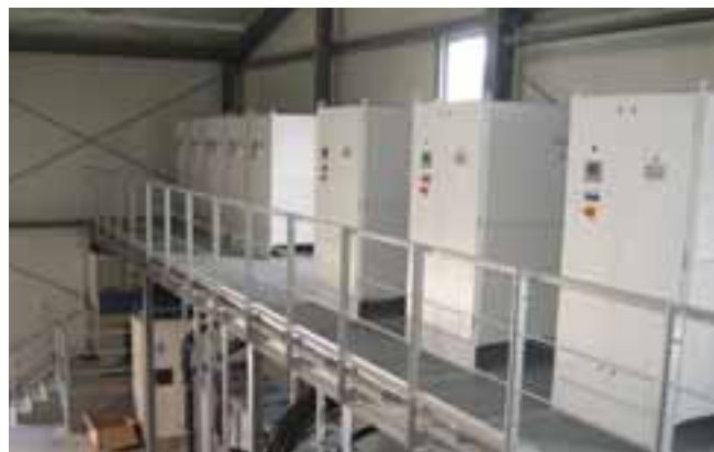
Fig. 7: Capacitive, inductive and resistive load units (from left to right)
