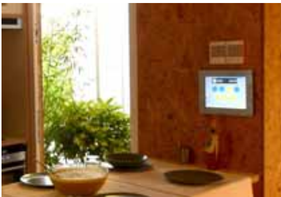
Fig.15: Building Control system and sensors
