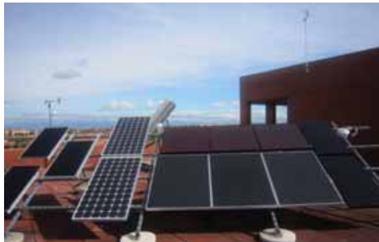
Figure 1: Outdoor PV facility installed in the University Carlos III de Madrid for testing the PV modules used in the study
