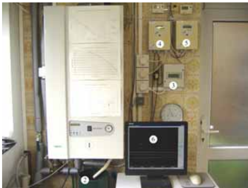
Fig. 2: 1 Boiler, 2 Rain Gauge, 3 Electricity sub-meter, 4 Heat Meter-Boiler, 5 Heat Meter-DHW, 6 Screen of Data Logger PC.
