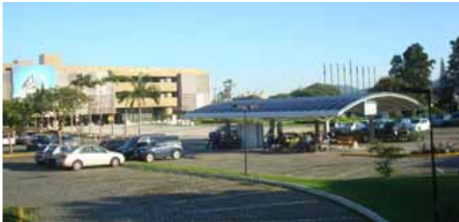
Fig. 2. Curved surface 11.97 kWp PV array integrated as a car port roof cover at the utility company ELETROSUL headquarter's building.
