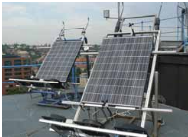
Fig. 4: Investigated unglazed PV-T collectors at test stand
