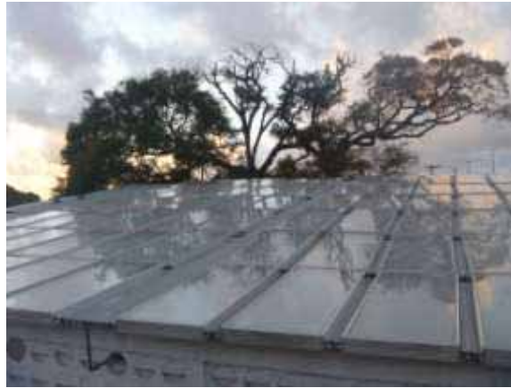
Fig. 1: Field of high efficient solar collectors installed in the LES/UFPB.
