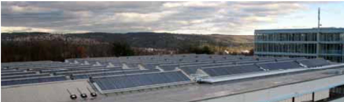
Figure 1.1: Foto of the Collector array of the solar air conditioning at Festo AG & Co. KG in Esslingen.
