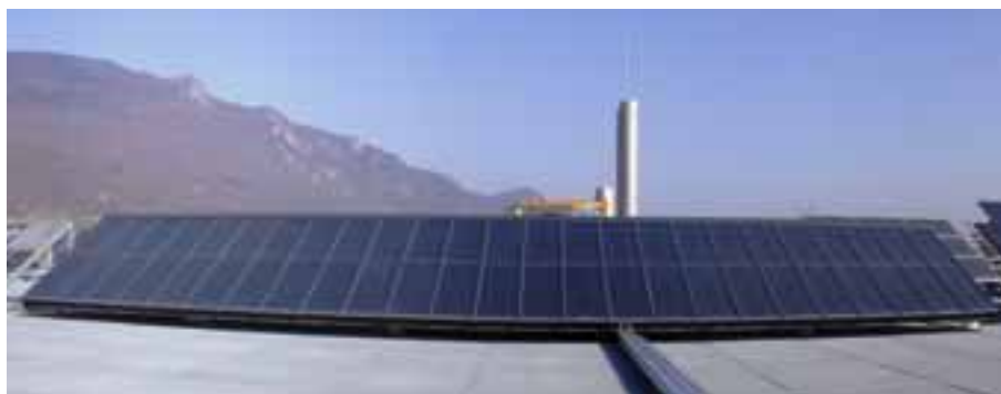
Fig. 3 : 30m² flat plate solar collector field on the top roof
