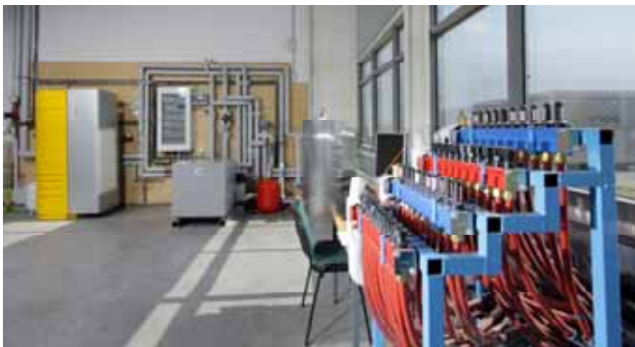
Fig. 5 : View of operating installation, absorption machine, cold storage tank and ground loop collector
