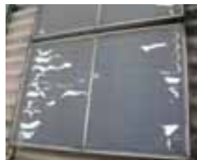
Fig. 16: Deterioration of paint
