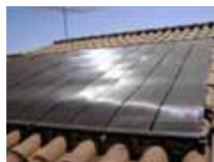
Fig. 24: Collector panels for solar pool heating
