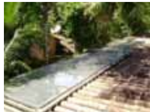
Fig. 20: Shading on the collector panels
