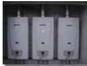
Fig. 11: Auxiliary heating system by gas
