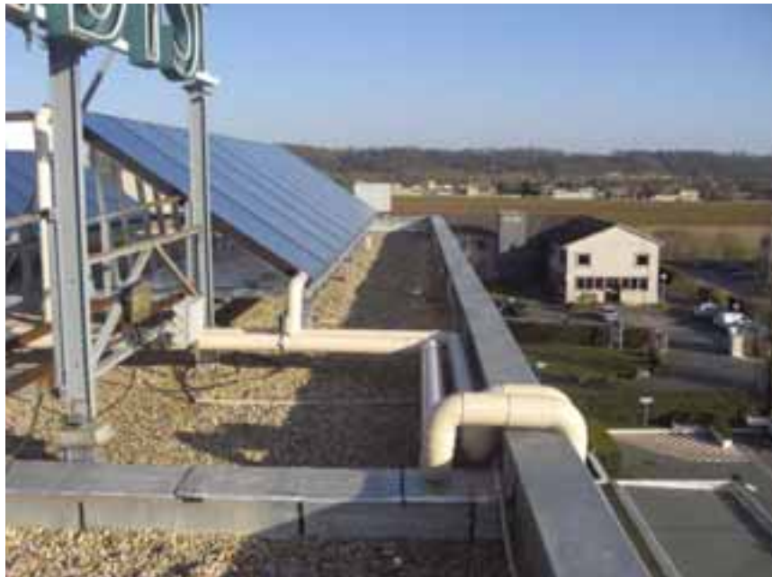
Fig. 4: Example of a « high point » case in the main piping connection in a drainback system for an hotel in Villefranche sur Saône (« high point » level lower than the one of the lowest part of the solar collector field)
