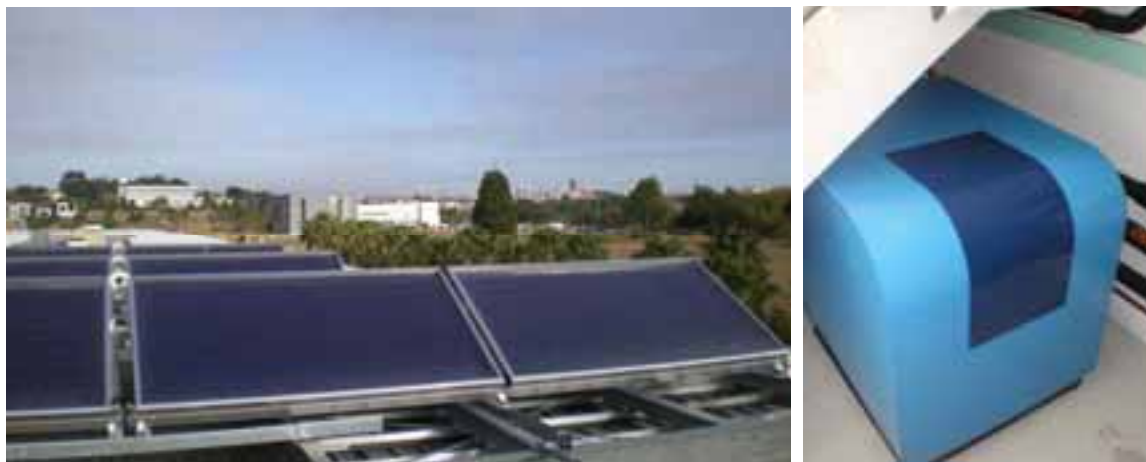
Fig. 12 : Double-glazed flat plate collectors and adsorption chiller installed at a laboratory/office building in Perpignan, France
