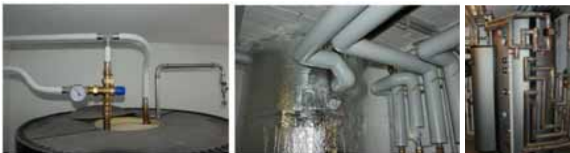
Fig. 8: Thermal insulation of heat store and connected piping, bad (left side) and good (middle) respectively well insulated with improvement by using thermosiphon breaks (right side); (Papillon et al., 2010)
