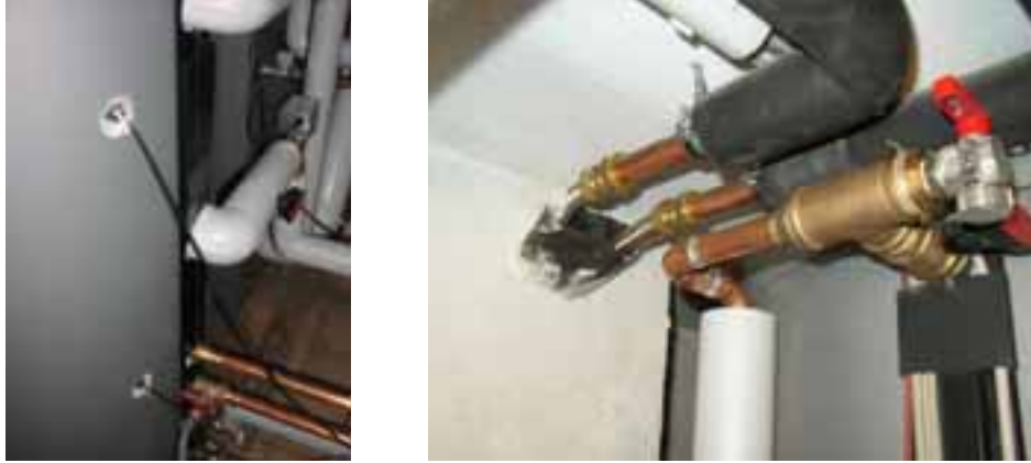
Fig. 2: Good (left) and bad (right) example for the thermal insulation at heat store connections
