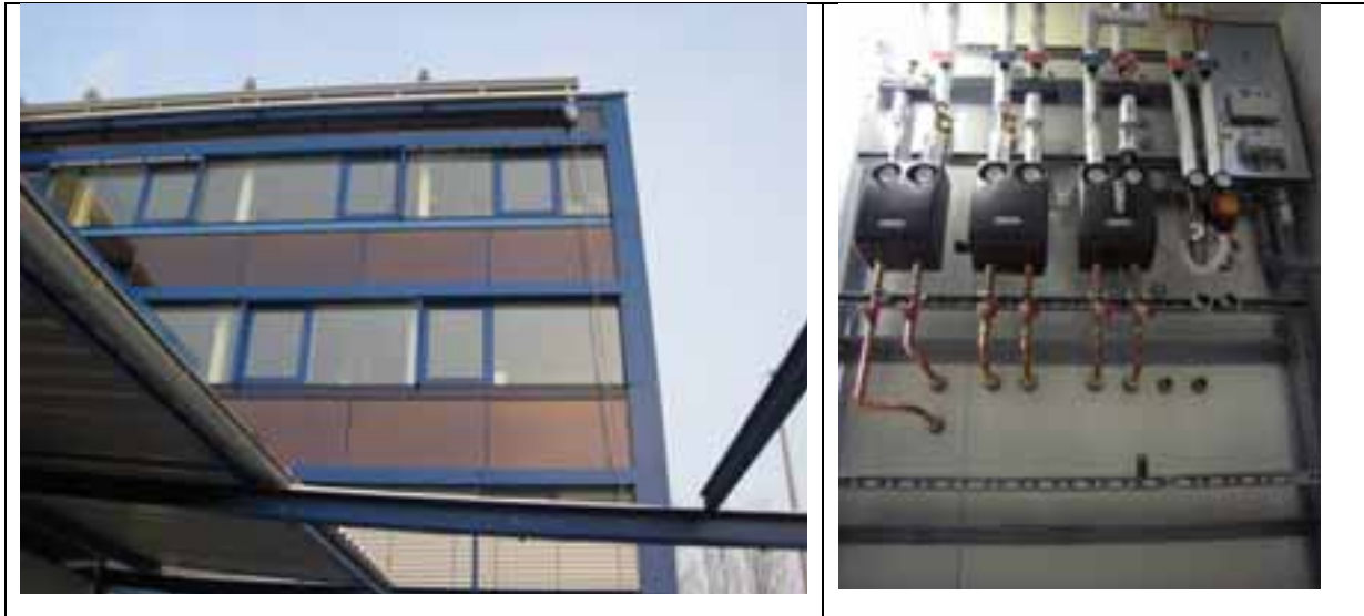
Fig. 1: Installed energy façade at the company site of Heinrich LAMPARTER Stahlbau GmbH & Co. KG (left) and installed heat buffer storage FLEXSAVE (right).
