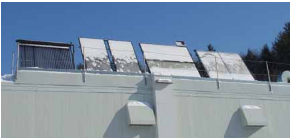
Fig. 4: Real winter conditions: solar panels covered with snow
