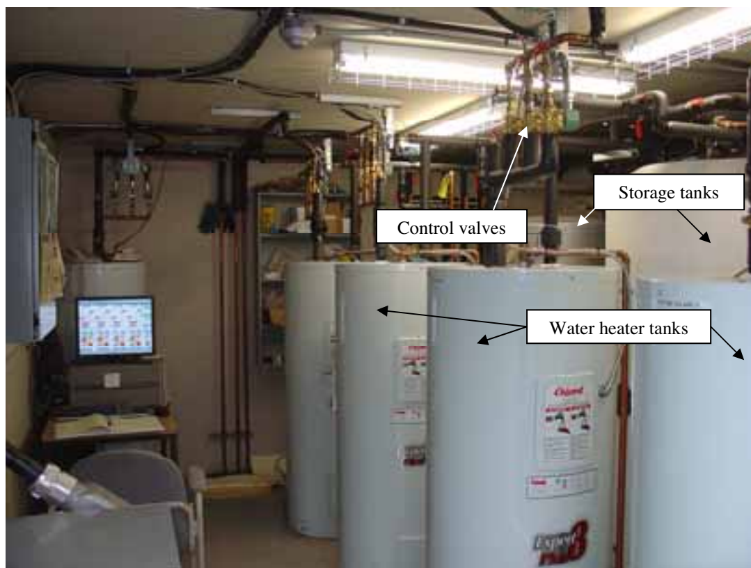
Fig. 2: Inside the annex: storage tanks, electric water heaters, control valves
