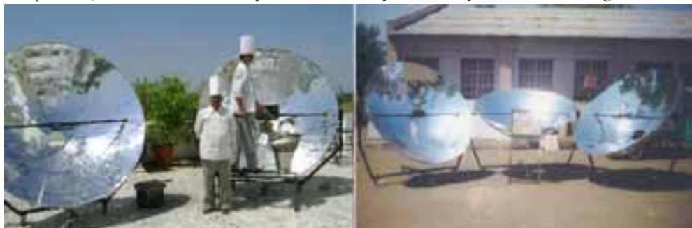
Fig. 1 Installation at Hotel Emerald Park Nasik and at a tribal school in Nandurbar district
