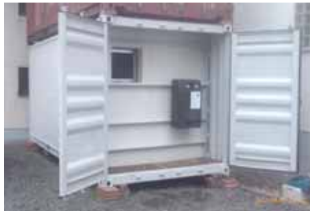
Fig. 5: Customized 20 feet marine container that serves as heat store.
